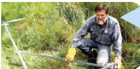
Tambo Bluff Landcare Coastcare volunteer installing the boardwalk to access the Middle Gully walking track.
